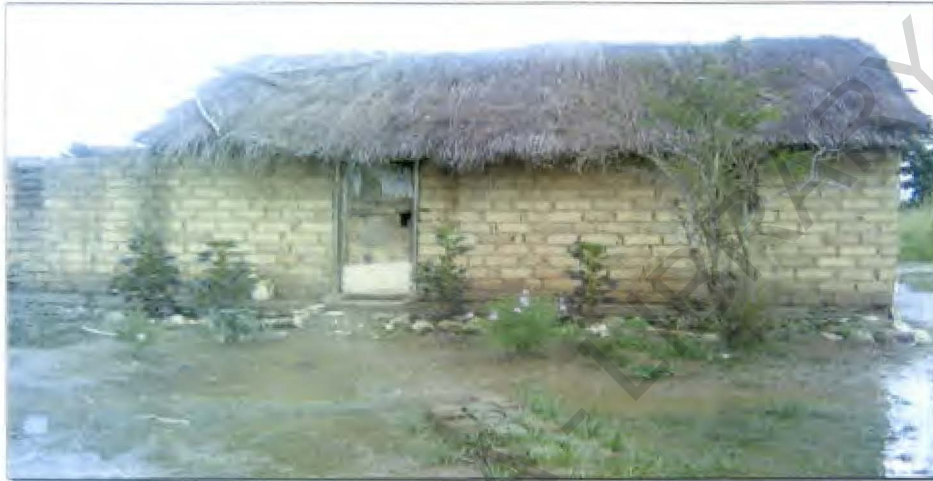
Photo 1: Destruction of Nehemiya's house by floods
