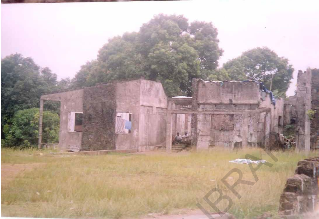
Plate 13: Houses destroyed during the war. Photograph by Bosede Awodola, (2006)
