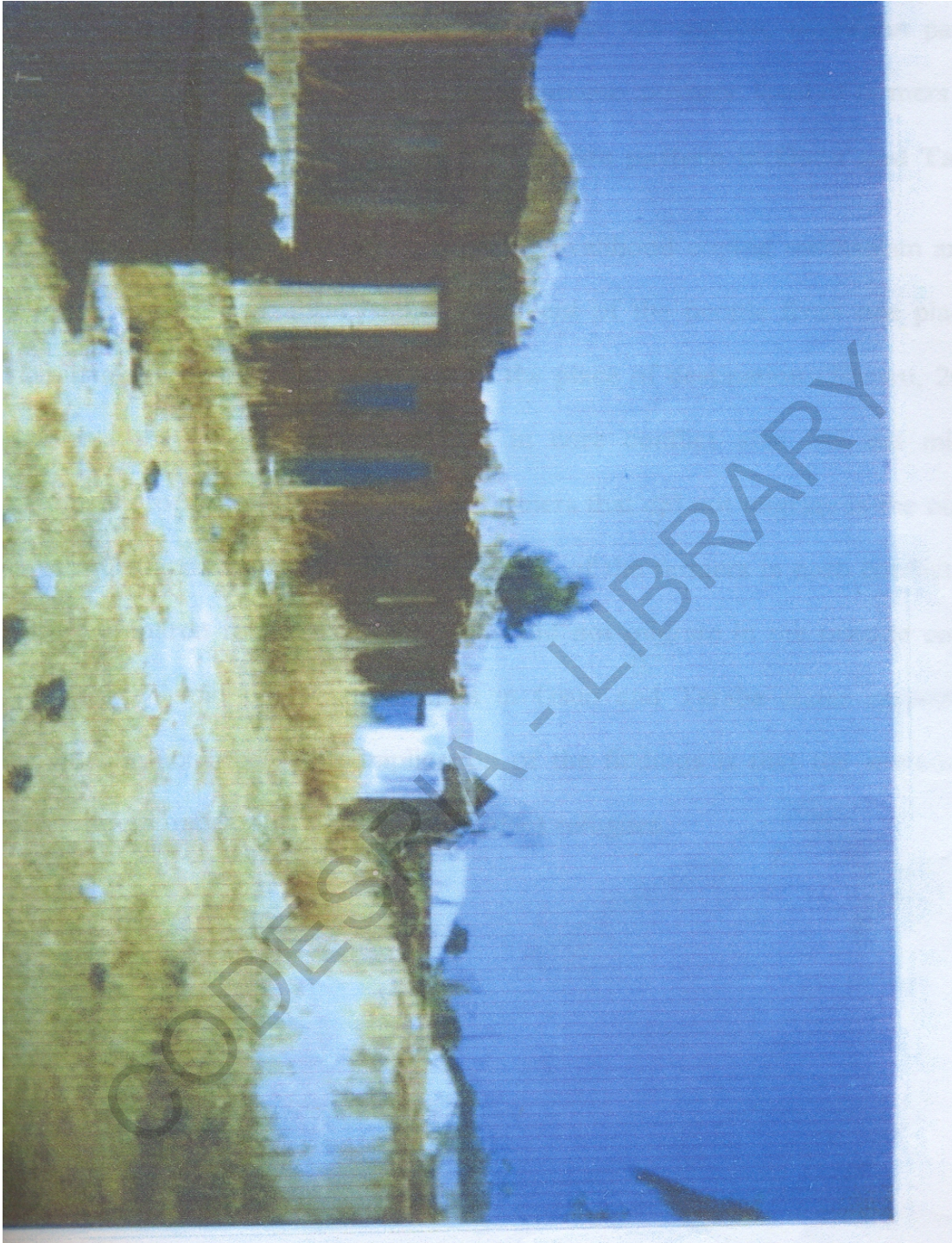
Plate 5.4: Vandalized Buildings in a farm settlement
