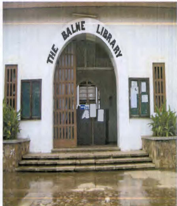
8. No access ramp at the main entrance of the Balme Library (the biggest on campus)
