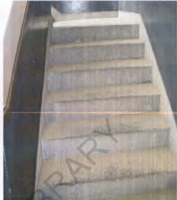
6. Several stairs leading to the office of the Coordinator of Disability services located on an upper floor without an elevator or lift
