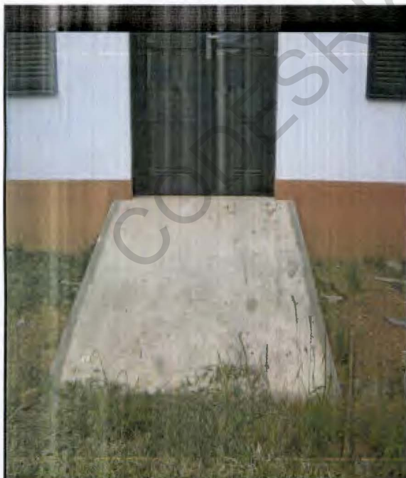
7. An accessible ramp constructed at the newly built east-wing of the Balme Library
