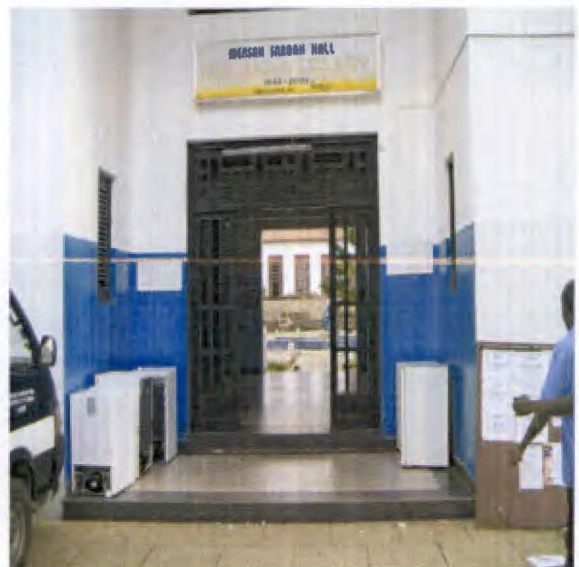
4. No accessible ramp at the main entrance of Mensah Sarbah Hall. A ramp would make the hall accessible
