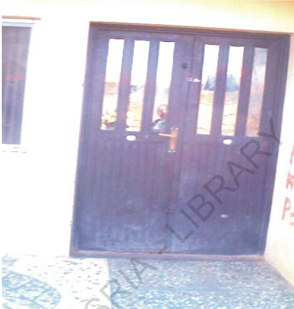
Plate 5.1: Steel door with a 'see through' glass in the low density residential area.
