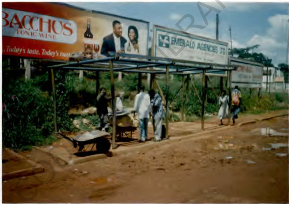
PLATE 2: Dilapidated Bus stop Shed.
