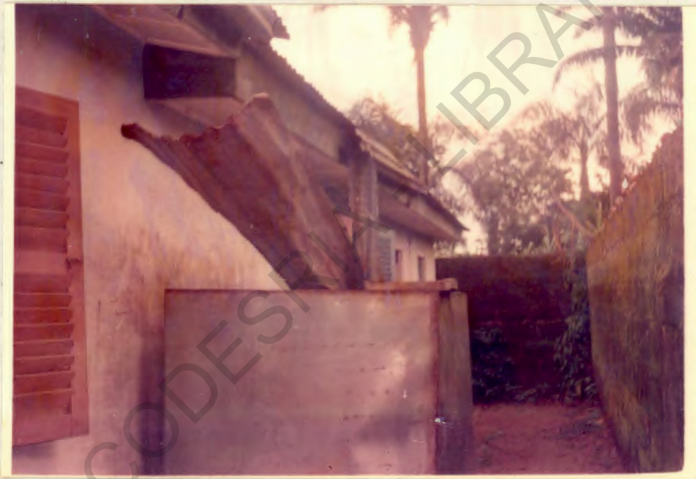
PLATE 10B: Corrugated iron eaves used to channel rainwater from the corrugated iron roofs to the storage tanks.
