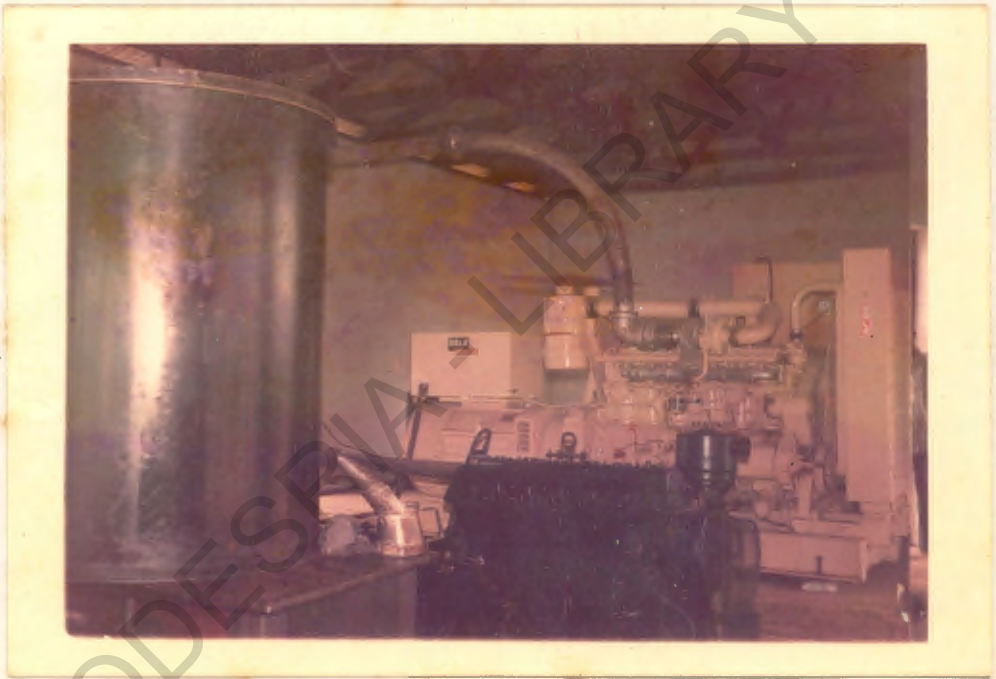
PLATE 5: A pumping plant of 159 kilo volt amperes (KVA). Every rural water works in the area has one of this type of pumping plant.
