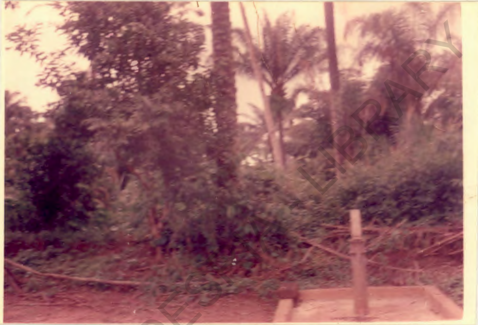
PLATE 12: A non-functional UNICEF mono-handpump in Umuogu village in Nsulu community.
