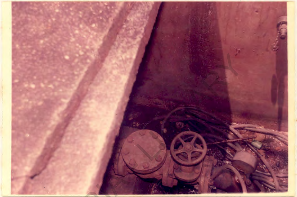
PLATE 4: The Nbawsi rural water works borehole at Umunkpeyi-Nbawsi. The borehole is protected with concrete slabs.
