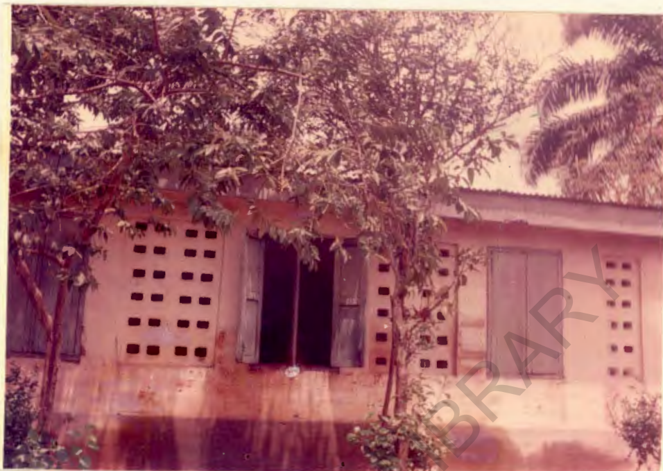
PLATE 6A: Eziama rural water works pump house at Eziama village in Nvosi community.
